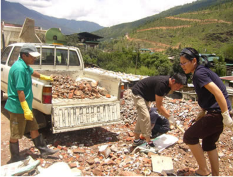
One of the members' Hilux used as pickup truck. We took the rubbles dumped near Drukonet (call center) to fill up the pot holes.
