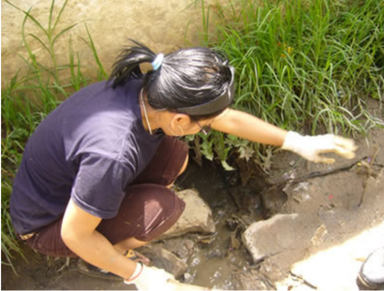
Cleaning the drain on the same road. This is the cause for the number of puddles on the road.
